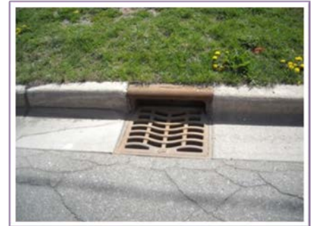
Unobstructed Catch Basin
